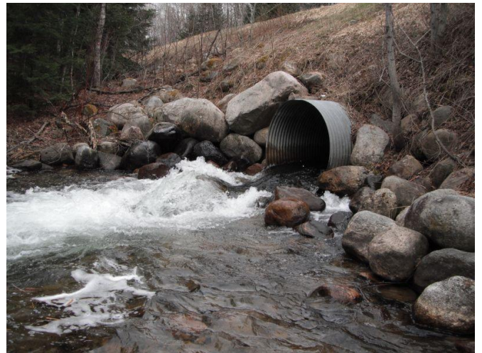
Photograph of the downstream view of the current culvert where the Wabana Creek passes under Route 49.
